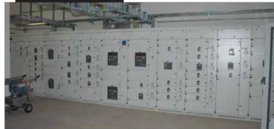
Power Center B.T. - Power Center B.T.
