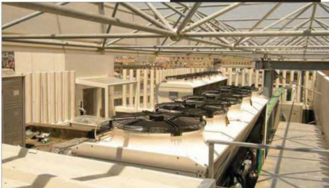
Centrali tecnologiche - Technological station
